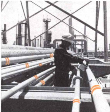
Workman is painting a section of Fibercast Pipe bearing 32% HCl at Shell's Texas Chemical plant. Note that Fibercast has sufficient strength for installation on span racks with the spacing normally used for metal pipes.
