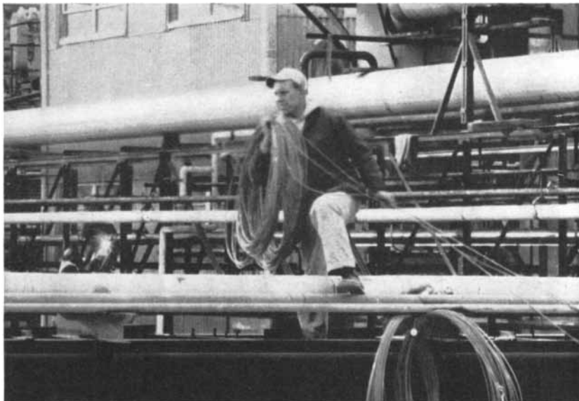
Installing PLASKON Nylon instrumentation tubing at Allied Chemical's Hopewell, Virginia plant. Note the 1000-foot, continuous, light-weight coils held by workman.
