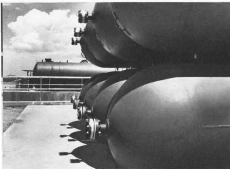
The Atlas is powered by a cluster of liquid propellant rocket engines that burn liquid oxygen and RP-1, a kerosene-like hydrocarbon fuel. 192 pressure tanks fabricated from alloy or Stainless Steel plate at this site store liquid and gases—liquid oxygen and nitrogen and helium gases which are used to inject the fuels into the missiles.
