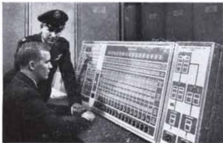
The Central Automatic Monitoring Console displays the status of the entire site, and displays equipment degradation prior to failure.
