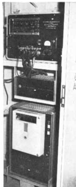
Clock, control unit, and recorder mounted in the Gyro Room of the Mormacpride's Bridge Deck.
