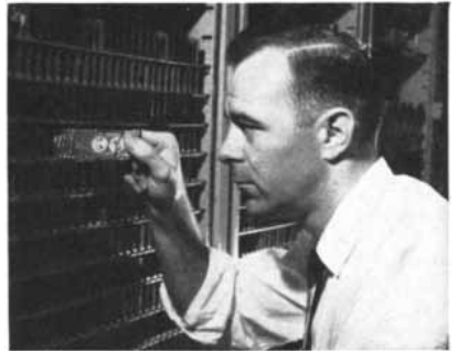
It was experimenting with an electronic central office at Morris, Ill., which is capable of providing a wide range of new telephone services.
