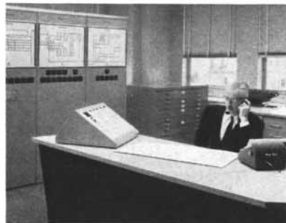
Heart of the system. Automatic data acquisition and display gives true "fingertip" control to dispatcher J. H. Philips, enabling him to distribute peak day-loads up to 750 million cubic feet of gas to Peoples' 275,000 customers.
