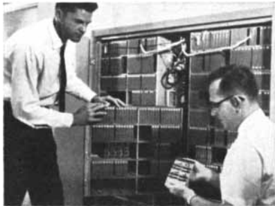
Holmdel Laboratory, N. J. We were developing an electronic switching system using new solid state devices. It will bring telephone customers a whole new range of services.
