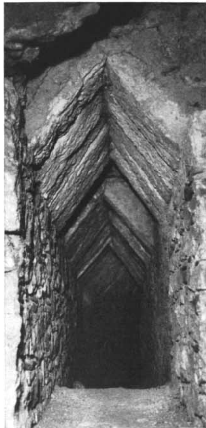
GABLED ROOF at the south end of the tunnel is characteristic of ancient Greek construction. The roof is made of pairs of large, flat stones leaning against each other.
