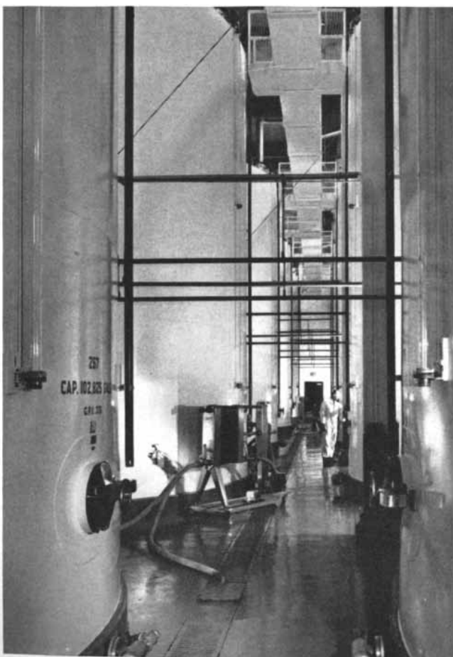
FERMENTING TANKS shown here can hold 100,000 gallons. They are made of concrete with a glass lining. The thin pipes between the tanks exchange heat to maintain a uniform temperature.
