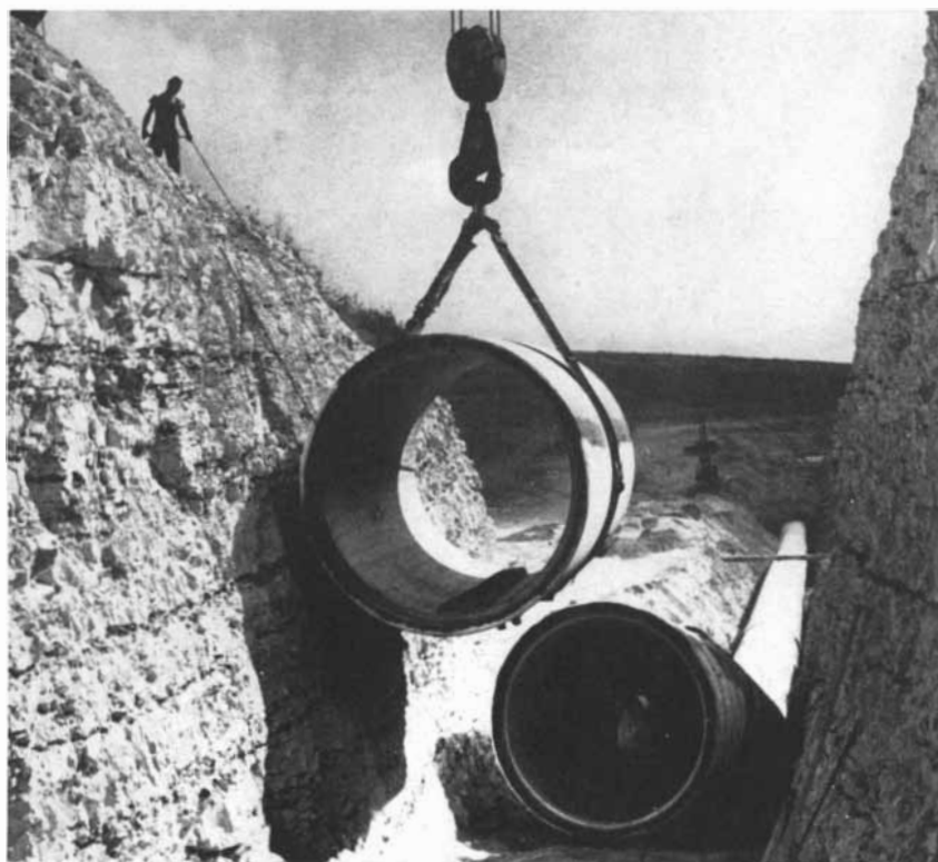
TRUNK-LINE PIPE , 108 inches in diameter, is laid by Israeli workmen. Israel's trunk line carries water from Lake Tiberias in a combination of canals, pipelines and tunnels.
