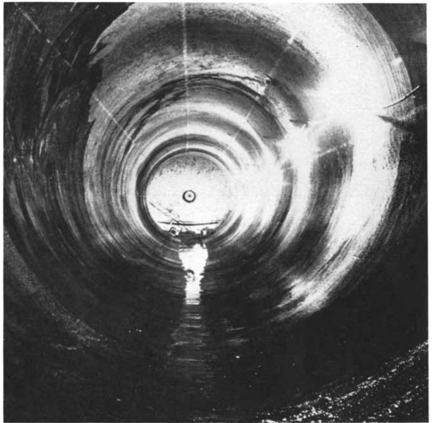
“CORRIDOR” TUNNEL might be bored through deep bedrock by hydraulic tunneling machines. This machine-drilled segment of a New York water conduit is 12 feet in diameter.
