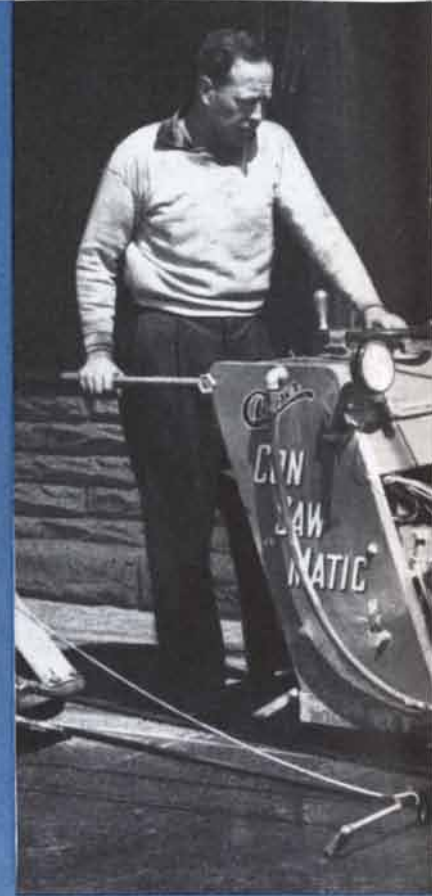
IN ST. LOUIS It was virtually necessary to "saw the city in two" by cutting over 20 miles of trenches down main thoroughfares for installation of underground lighting cables. Job was accomplished with natural-diamond blades cutting through concrete with gravel aggregate. Depth of cut: 1½ inches.
