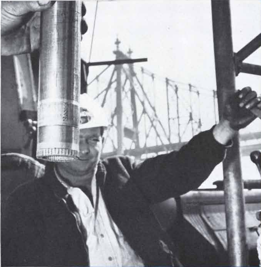
IN NEW YORK Test-boring along the route of a proposed subway tunnel under the East River was required to determine the composition of the rocky riverbed. Diamond drill bits driven from a barge platform in 85-foot-deep water are recovering core samples 2.155 inches in diameter.
