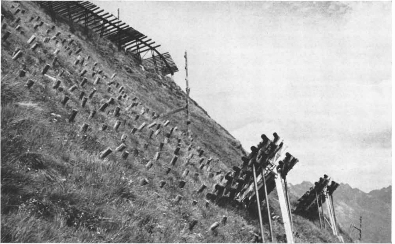
EXPERIMENTAL INSTALLATION on the Dorfberg at Davos is aimed at providing support for a body of snow and hence deterring avalanches. The two lower structures have instruments to measure the pressure of the snow. Effects of the pressure are re-
