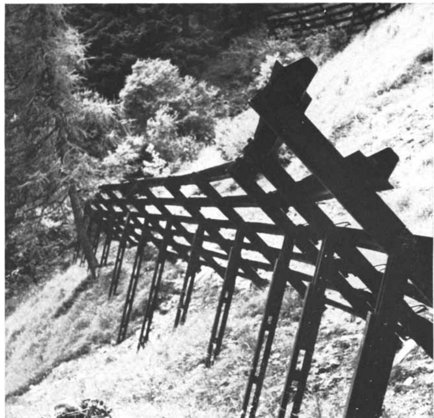
AUSTRIAN STRUCTURE was designed to prevent the formation of avalanches by helping to anchor snow. Made of steel and about 10 feet high, it is located near the Brenner Pass.
