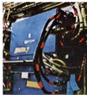
IBM computer and data adapter installed in the Instrument Unit.
