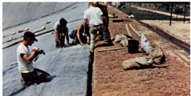
Rubber surface is anchored in a shallow trench dug around edge of reservoir. Trench is then filled and tamped.
