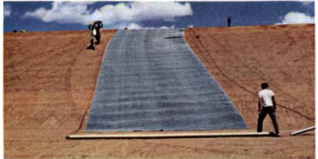
Royal-Seal rubber surfaces are easy to install. First step is to unroll the 20-foot-wide rolls.
