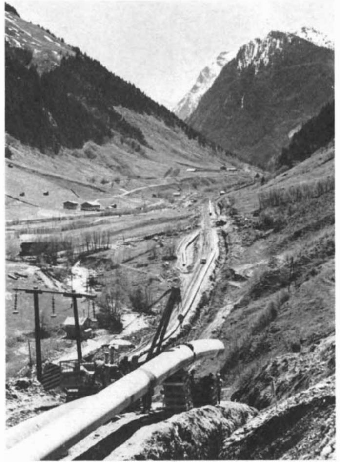
TRANSALPINE CONSTRUCTION of a 40-inch oil pipeline entailed special construction problems. Here the line descends into an Austrian valley north of a tunnel that is line's highest point.
