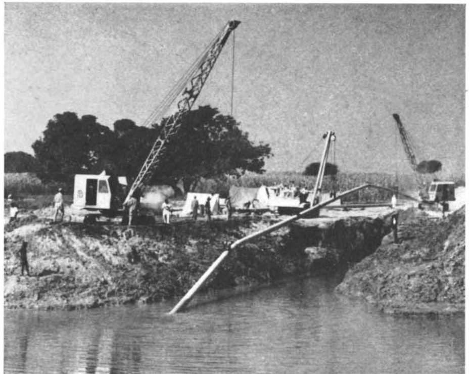
SUBMERGED CROSSING of a river is one of 77 being made for a 738-mile oil pipeline in India. The Bechtel Corporation, a U.S. engineering firm, is supervising the construction.
