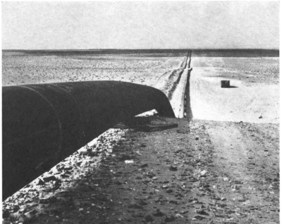
DESERT PIPELINE in Libya awaits coating and wrapping before being lowered into the trench. Desert construction requires special measures to keep the trench from collapsing.
