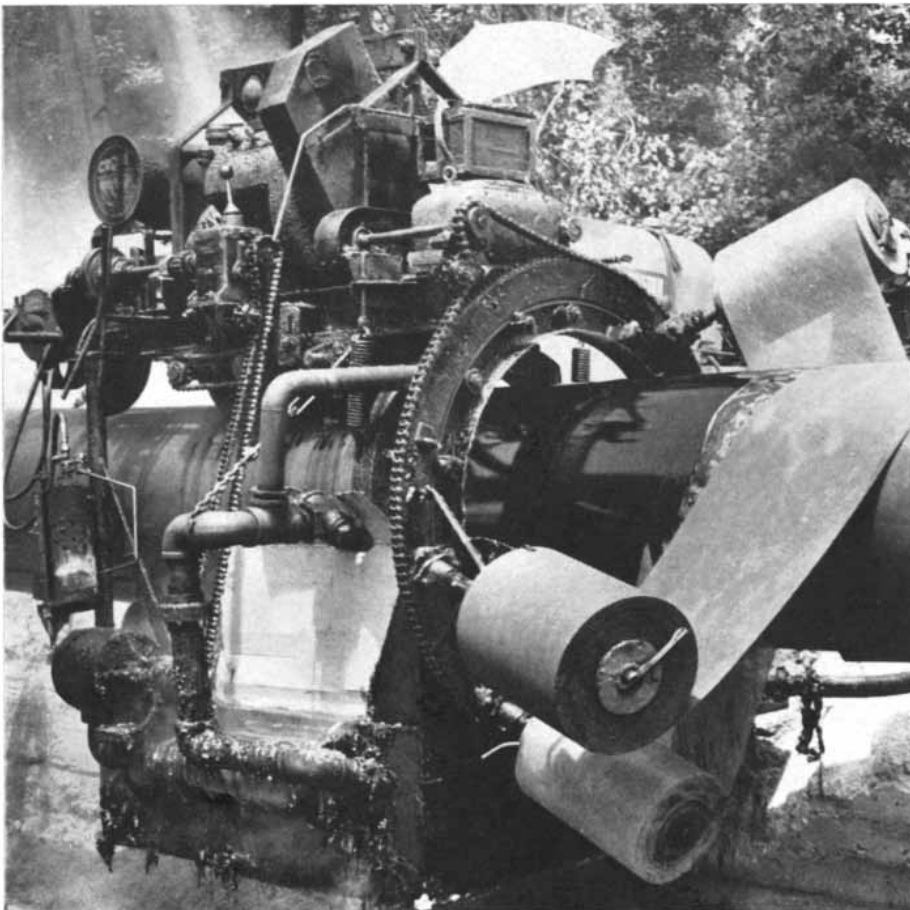
COATING AND WRAPPING of a pipeline is typically done automatically by machines such as this after the line has been welded but before it is lowered into the trench and tested.
