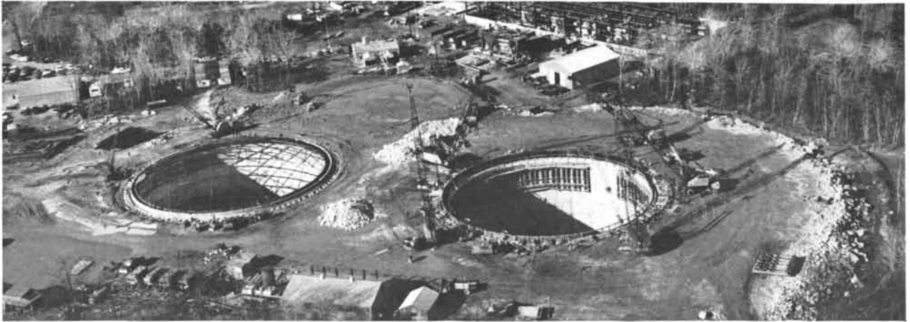
STORAGE FACILITY at the liquid natural gas plant of the Tennessee Gas Pipeline Company in Hopkinton, Mass., involved excavating two cylindrical pits, each 172 feet deep and 135 feet wide.
