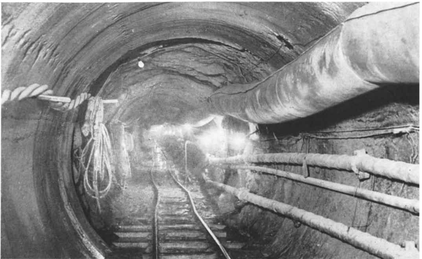
MACHINED TUNNEL was made in St. Louis by a continuous tunneling machine. The smooth wall in the foreground was produced by the machine; the rougher walls in the background are in a por-
