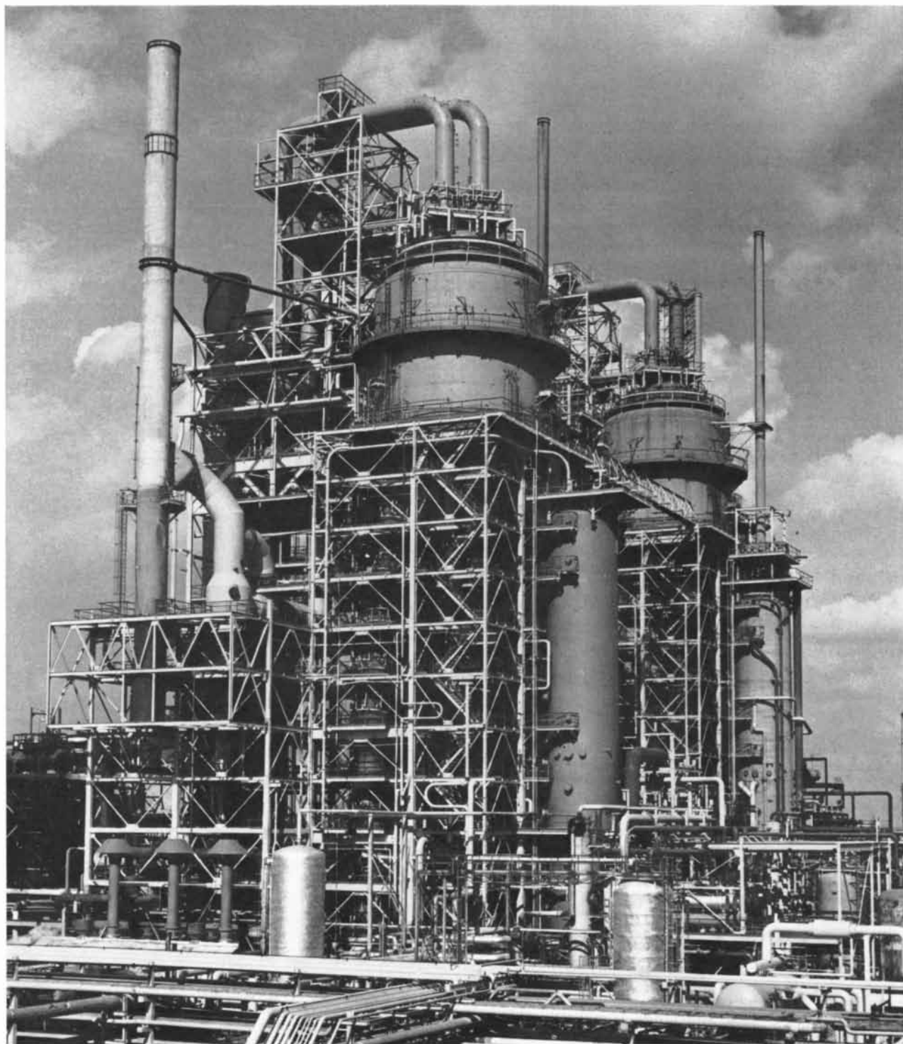
PETROLEUM CRACKERS using the fluidized-bed technique are operated by the Humble Oil & Refining Company in Baton Rouge. Two crackers are shown here. In each case the cracker and regen-
