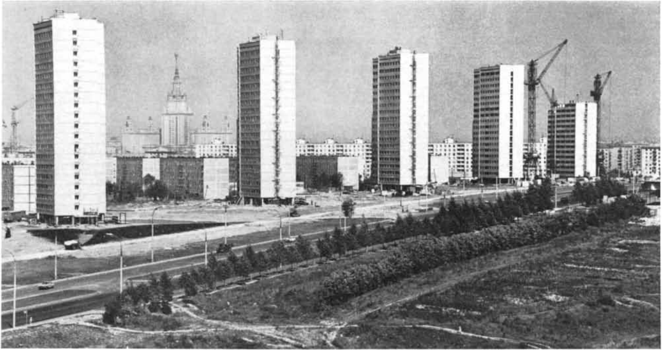
APARTMENT AND OFFICE BUILDINGS are under construction along Kalinin Avenue in Moscow. Nonresidential construction
