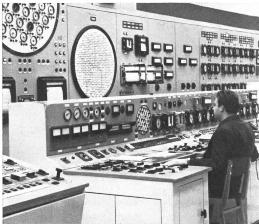
ATOMIC POWER CONTROL ROOM in Novo-Voronezh regulates a water-cooled reactor of 365,000 kilowatts. The U.S.S.R. placed the first atomic power plant in operation in 1954.
