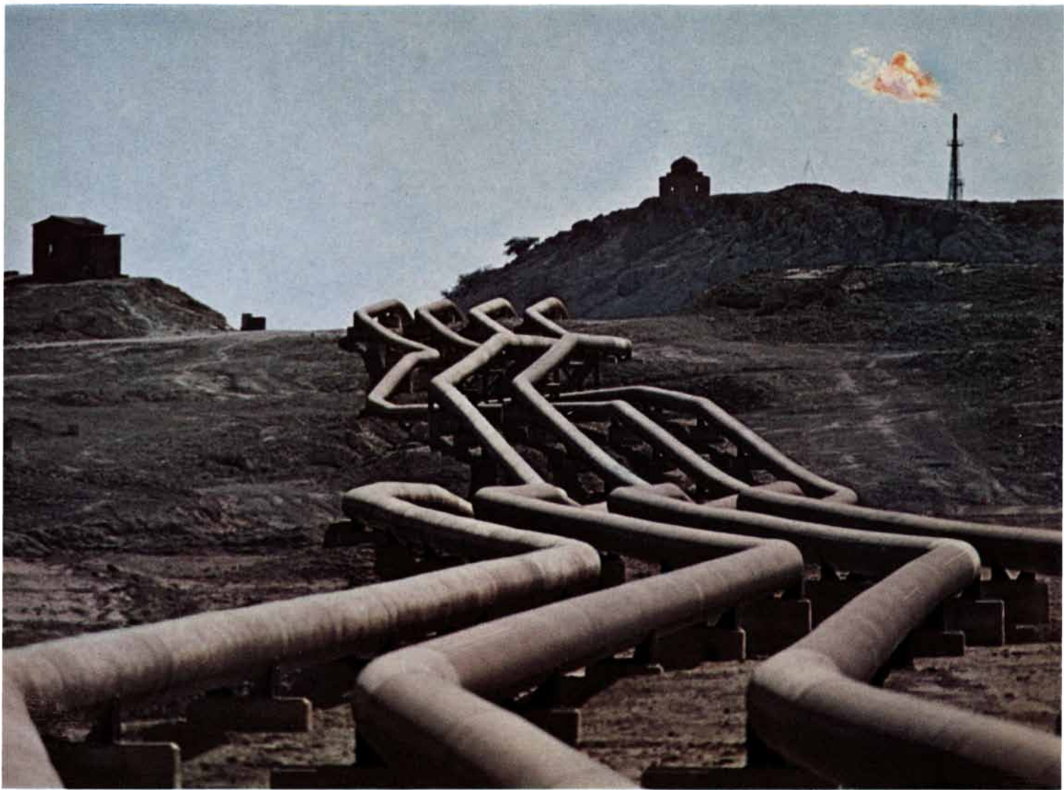
Standard Oil of N.J. terminal facility, Kharg Island, Persian Gulf.
