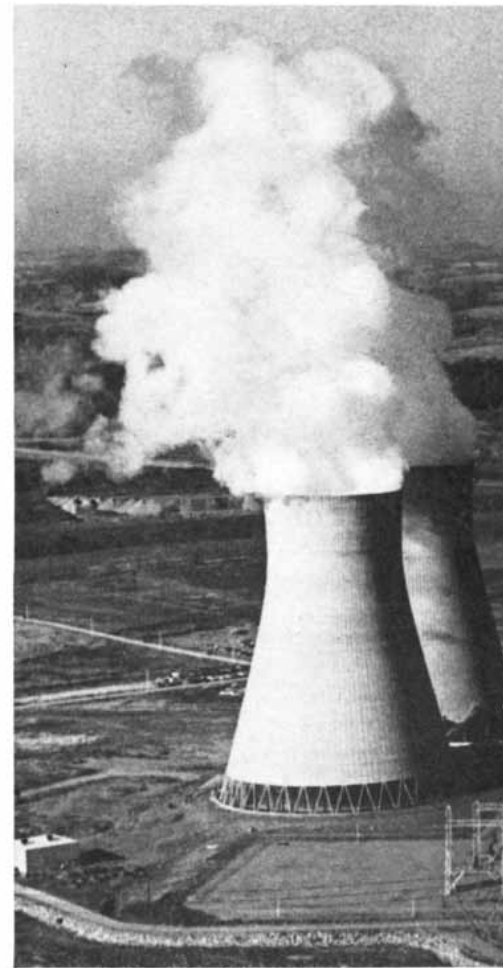
FOUR COOLING TOWERS serve the Keystone Steam Electric Station in western Pennsylvania. Each pair of towers serves one of the station's two 820,000-kilowatt gen-
