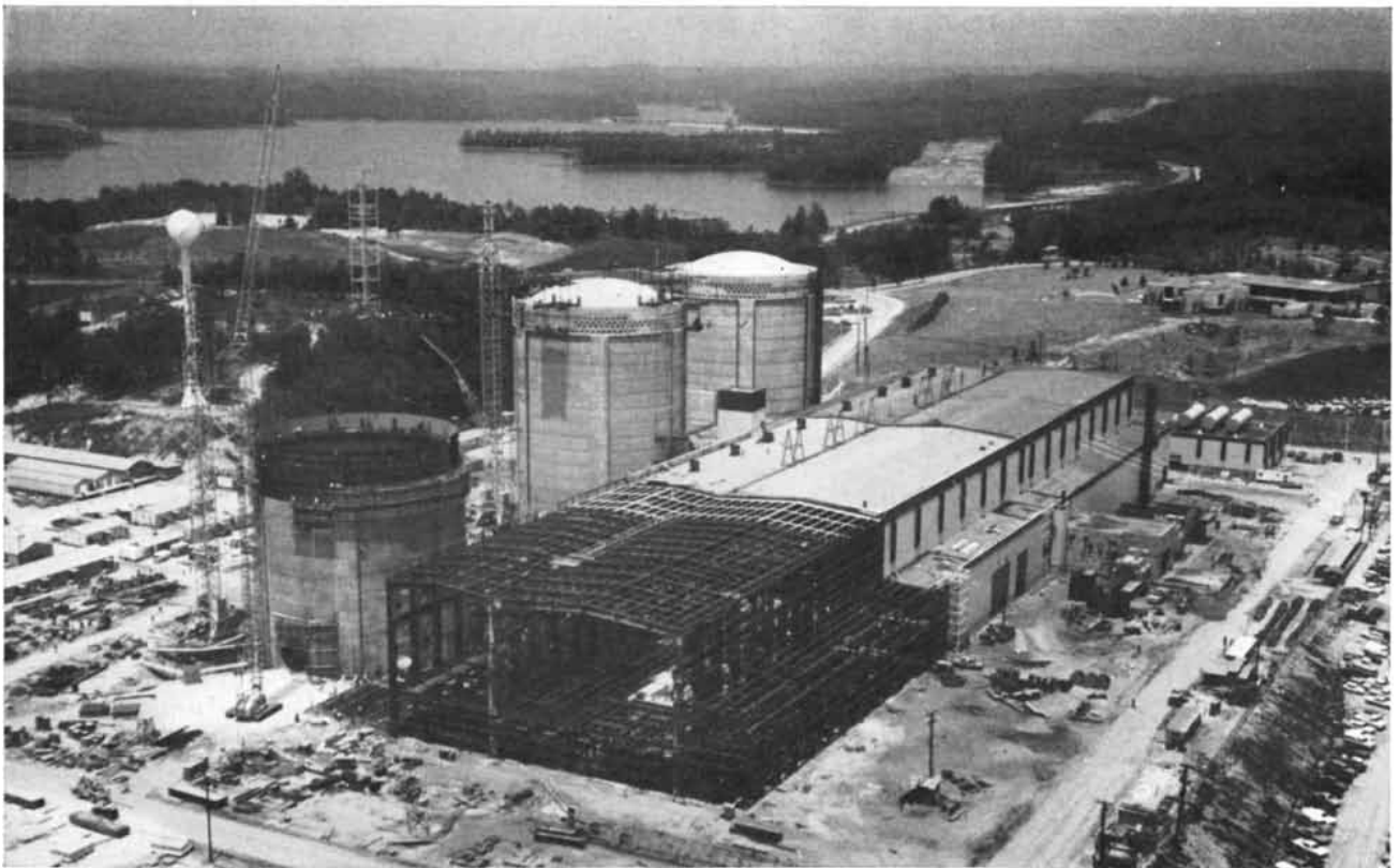
NUCLEAR POWER PLANT being built by the Duke Power Company near Clemson, S.C., has three 886,300-kilowatt units in various stages of completion. Unit No. 1 (right) is ready to be loaded with fuel; it is expected that it will be supplying power early next year. The three nuclear steam-supply systems were designed and are be-
