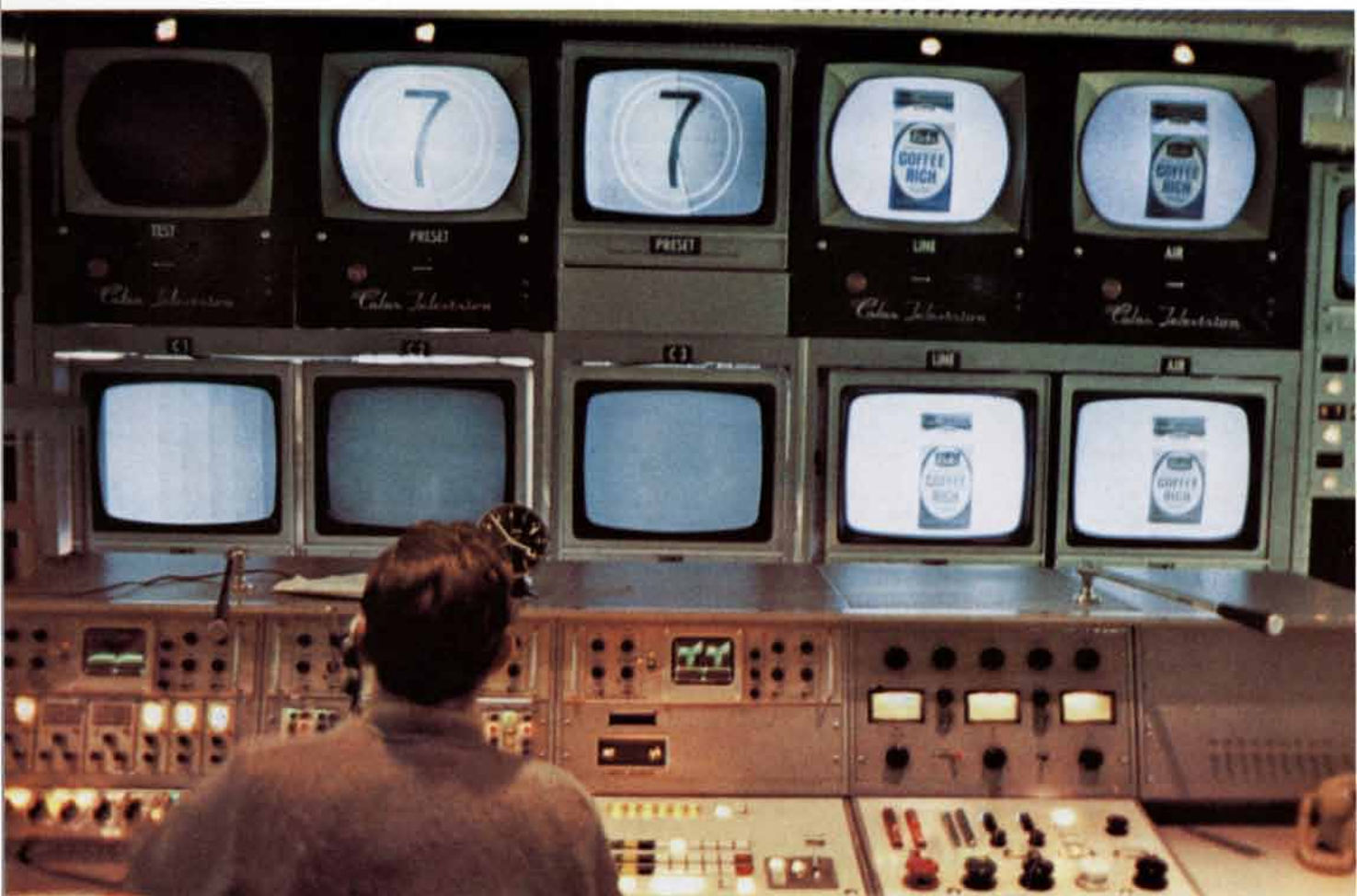
TV STATION MASTER CONTROL ROOM
