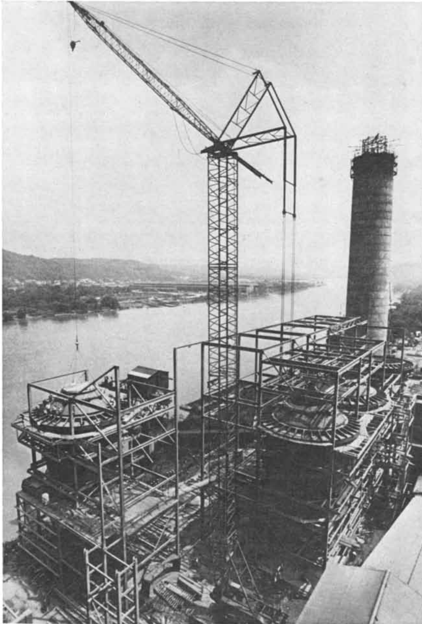
POLLUTION-CONTROL EQUIPMENT is installed at the Phillips Power Station of the Duquesne Light Company near Pittsburgh. The installation was in progress when the photograph was made. The three cylindrical structures at right are fly-ash scrubbers. The cylindrical structure at left is a sulfur dioxide scrubber designed to operate in conjunction with one of the fly-ash removers. The coal-fired plant has six steam generators and a total electrical output of 400 megawatts. The river flowing past the power plant is the Ohio River.
