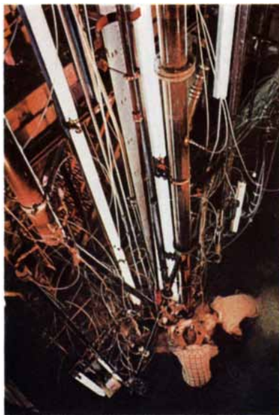
At Exxon's pilot plant in Baytown, Texas, various American coals are being converted into cleaner burning synthetic gas.
