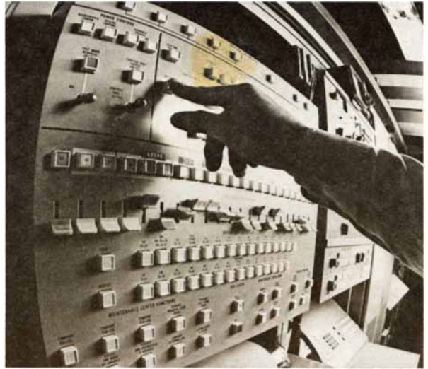
Electronic switching systems, a thousand times faster than the equipment they replace, are now being installed across the nation.
