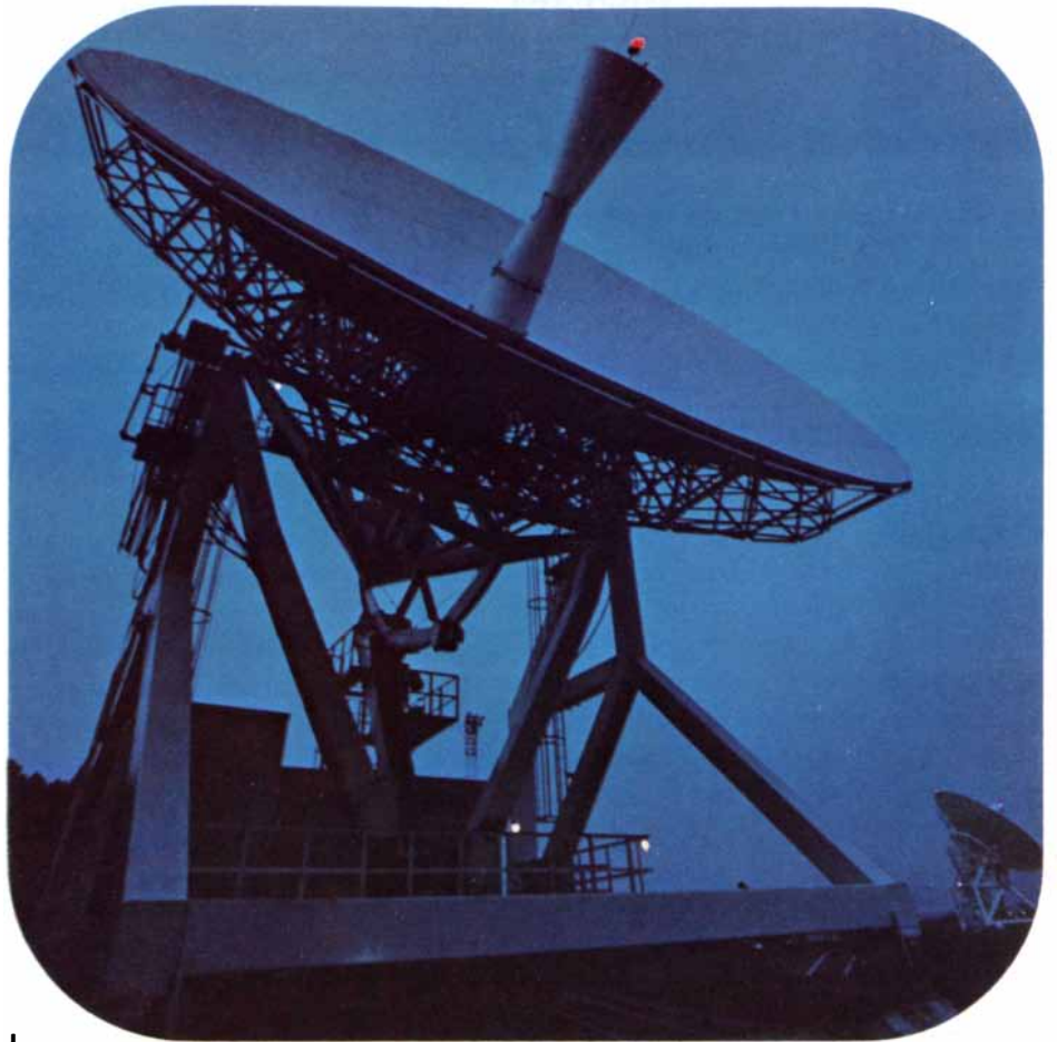
Harris Satellite Communications Terminal
