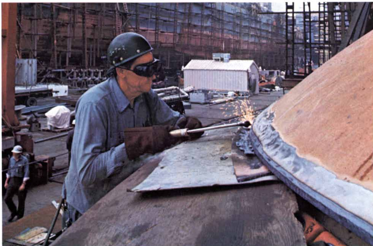
This welder at Ingalls Shipbuilding, has access to an IBM computer to verify that his construction drawings are up to date. Workers and engineers throughout the huge shipyard access a wide range of computer applications through nearby terminals.
