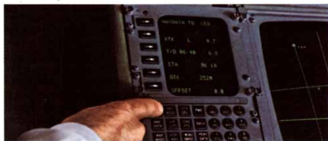
Flight management control panel.
