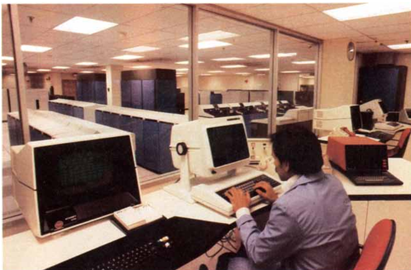
Computer banks at Mead Corporation's Mead Data Control Computer Center near Dayton provide storage and processing for on-line full-text information systems. LEXIS and NEXIS. Users easily access the base from remote locations through Mead-marketed interactive terminals similar to that shown.
