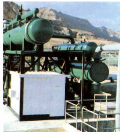
The solar electric power generating station at Ein Bokek
