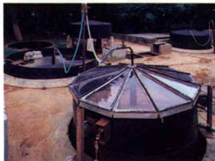
Improved experimental biogas plant with solar collector for family use.
