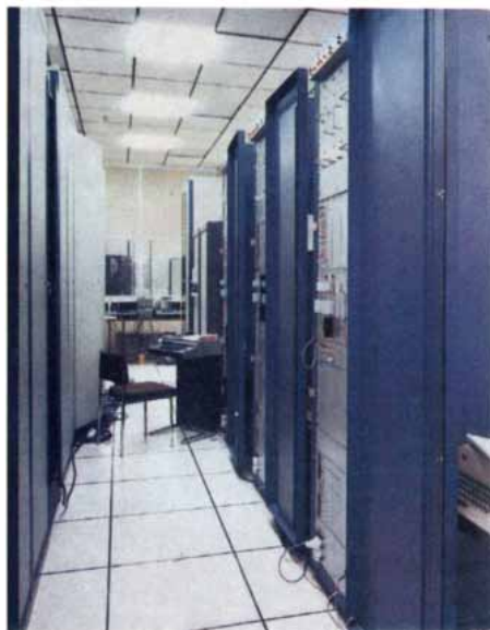
The Transpac packet-switched data network, with its operational center in Rennes, provides access to computers from remote terminals with tariffs independent of distance.
