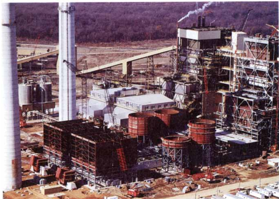
Fläkt's DRYPAC system is being employed at the Grand River Dam Authority's coal-fired power station near Pryor, Oklahoma.
