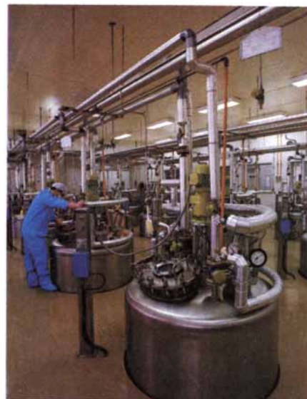
Typical fermentation plant
