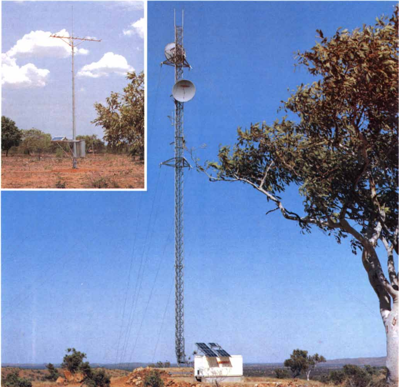
Solar powered microwave repeater station in remote NW Australia
