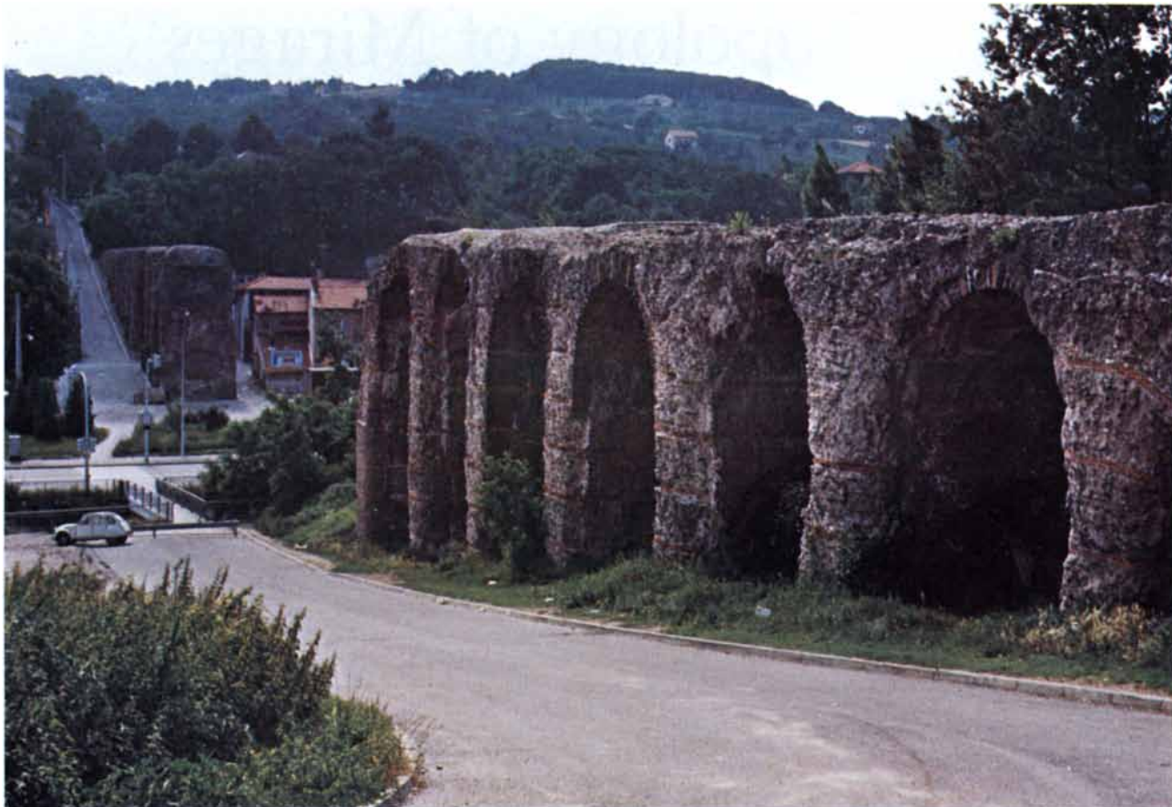
BEAUNANT VENTER is shown from the point (rear) of the first geniculus , where the pipes emerged from the ground and started across the floor of the valley. The venter was much wider (seven me-
