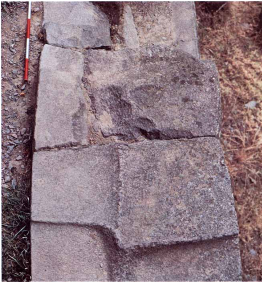
DISMANTLED INCA WALL at Ollantaytambo yields clues about how the Incas fitted stones. Each concave depression marks the place where a stone has been removed. The depressions were pounded out to precisely match the convex bottom surface of the upper stone.
