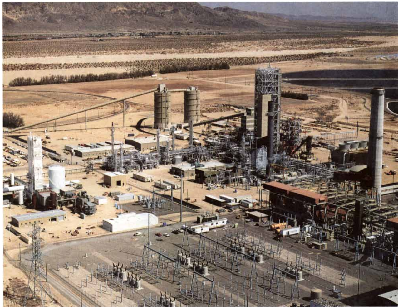
COOL WATER DEMONSTRATION PLANT of the Southern California Edison Company converts 1,000 tons of coal daily into a clean-burning gas whose combustion products drive a gas-turbine generator. The "waste heat" in the exhaust from the gas tur-
