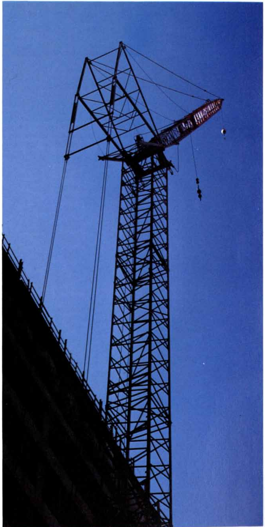
MOBILE CRAWLER CRANE with tower boom is lowering its hook to the ground, where it will receive a bucket of concrete for the concrete-framed building beside it. The building, photographed when 12 stories tall, will stand 45 stories when it is completed.
