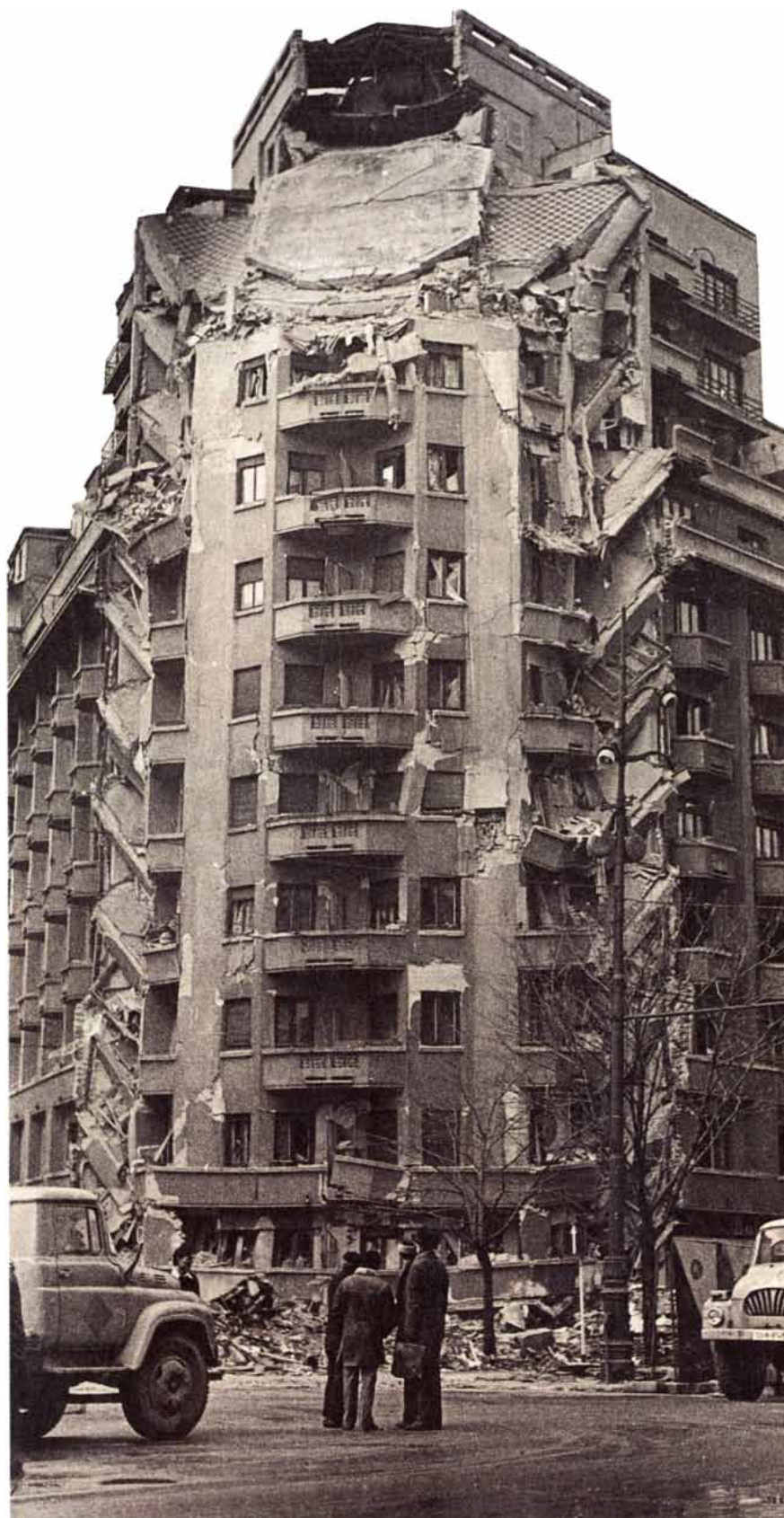
DESTRUCTIVE DEEP EARTHQUAKE is a rare event. The only severe one in recent decades took place on March 4, 1977, 150 kilometers under Bucharest. Columns on the ground floor of this building failed, allowing the corner to slump by one floor. Similar destruction throughout the city killed 1,500 people. The photograph was made by Neculai Mandrescu of the Institute for Physics of the Earth in Bucharest.
