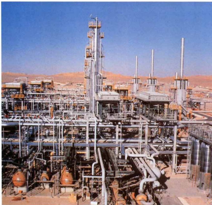
Natural gas treatment plant at Rhourde Nousse (Algeria)
