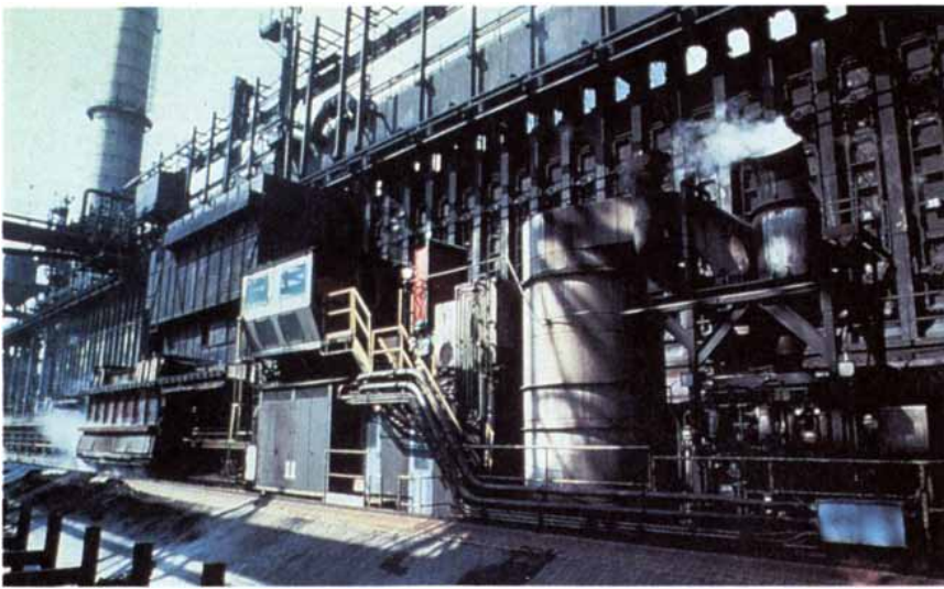
COKE-OVEN BATTERY (in background) burns coal in the absence of oxygen to produce coke. When the vertical panel doors are removed, coke is pushed from the battery into railcars. Scrubbing equipment (in front of battery) helps to control pollution. Photograph courtesy of the American Iron and Steel Institute.
