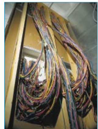
NETWORK CABLE: about 10 miles' worth in total.
