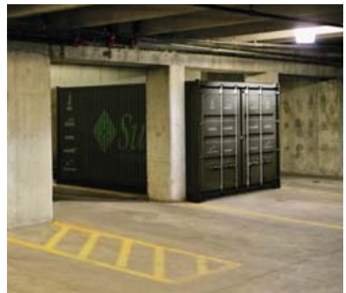
PARKING GARAGE could be the low-cost site for a company's new data center—if an Ethernet link and a water supply were available.
