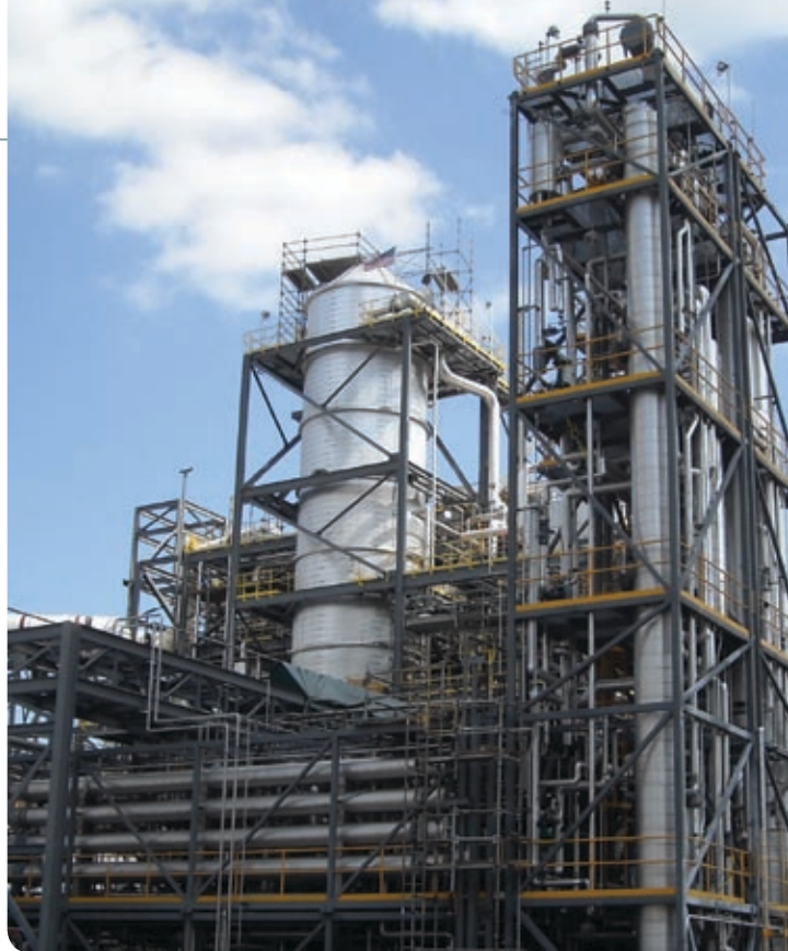
CARBON CAPTURE UNIT at the Mountaineer power plant near New Haven, W.Va., uses chilled ammonia scrubbers to grab carbon dioxide from coal burning for subsequent storage underground.
