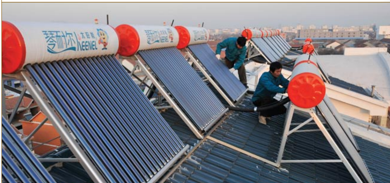
SOLAR WATER HEATERS are installed on thousands of rooftops in Rizhao, China, reducing electricity demand for domestic hot water.
