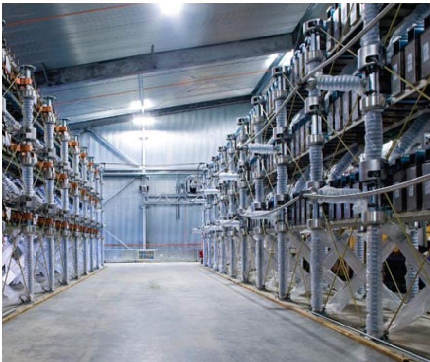
Massive electronics convert alternating current to direct current for Trans Bay Cable's 53-mile, high-voltage line that runs along the bottom of San Francisco Bay.
