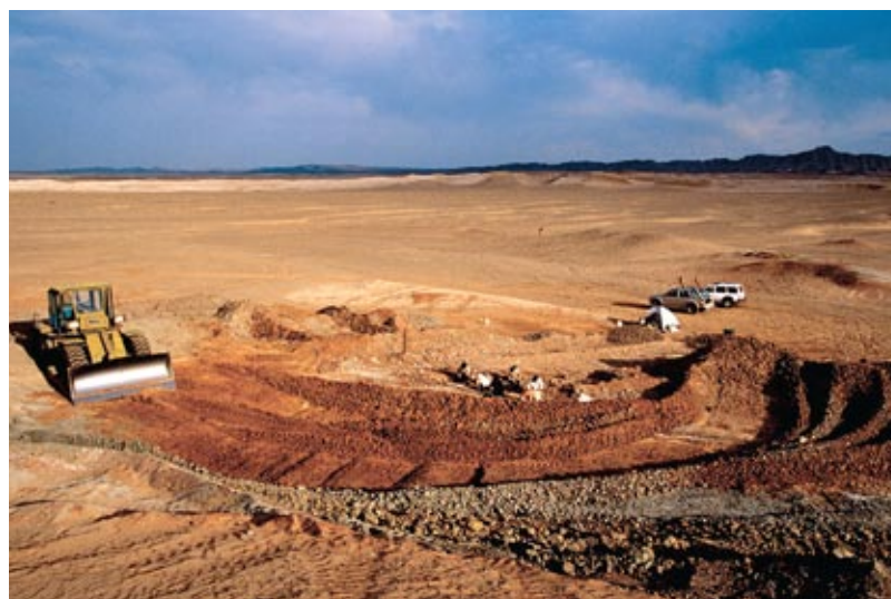
Speed the plow: Without this bulldozer, on loan from a nearby Chinese army base, the excavation would have taken months, not weeks.
