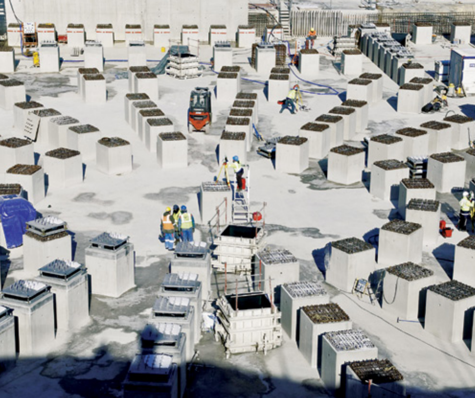
SOLID FOUNDATION: The reactor will sit on 493 columns topped by steel-and-rubber bearings to isolate the 400,000-ton structure from seismic vibrations.
